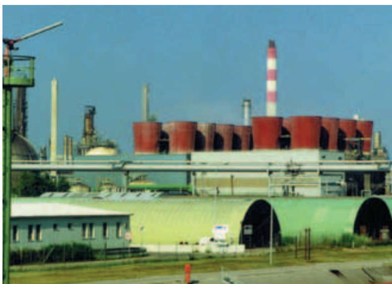
Cooling Tower at OMV, Vienna
